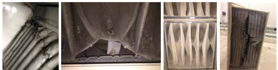
Figure 2: Common filter failures in air-handling units (media rupture, disintegration, deformation, fracture)
